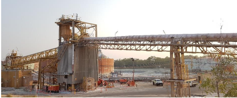
$4.5M – QAL replaced an alumina conveyor with a sealed airslide, eliminating airborne alumina during transfer at this point
