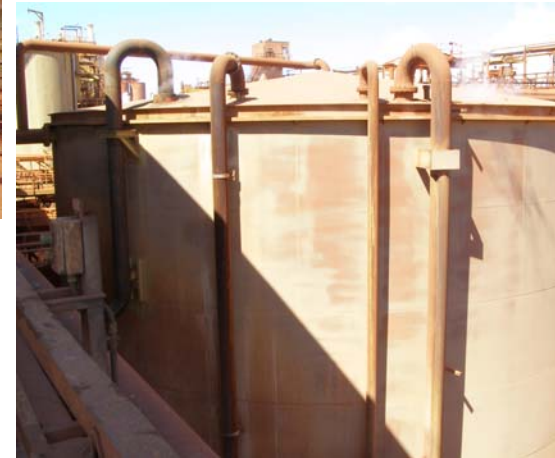
Wash water tanks
